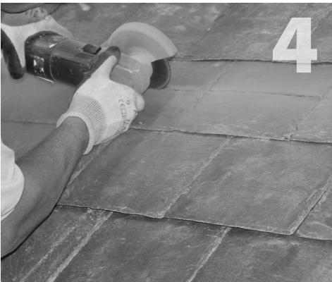
Using a cutoff wheel in a grinder, score the slate above the mounting area at 4 inches above the center of the QBase location. In step 5, you will remove the slate below the score line, which will allow you to slide the flashing up under the remaining slate in step 10.
