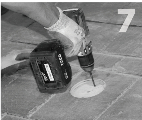
Using QBase (item 2) as a guide, align two clearance holes vertically with the center of the rafter. Mark the center of these 2 holes. Drill 7/32" pilot hole at each of the 2 marks. Hold drill square to rafter. Do not use QBase as a drill guide.
