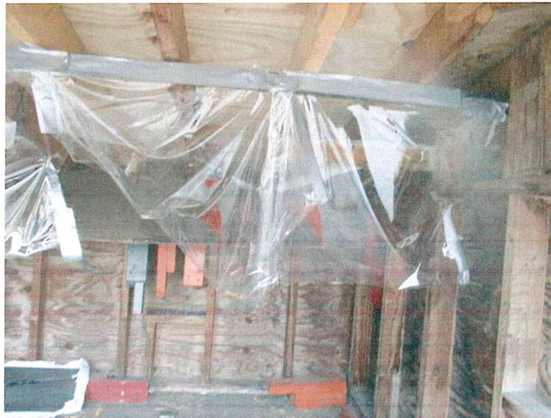
Photo No. 10 Underside of Test Specimens #3 and #4 After Testing
